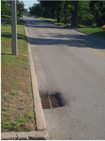
Above: Looking North on Flood at the southbound lane, sunken grate on west side adjacent to Lions Park and the concrete lined stream channel.
